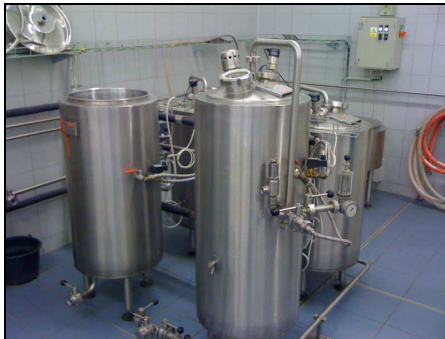
Figure 1: Fermentation part of Destila micro-brewery assembly. Note the cylindroconical fermenter in the foreground with extensive piping accessory (position of SENSOR2). Photo by D. Varner
